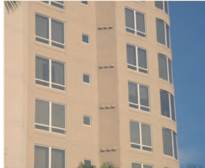
PHOTO 4 Lots of Penetrations. You want energy efficiency? You want a controlled indoor environment? You want to build tight and ventilate right? You better get used to living with the holes. Putting the stuff on the roof or at the bottom of the building does not work. Might work in houses and row houses and town houses, but not in apartments.
